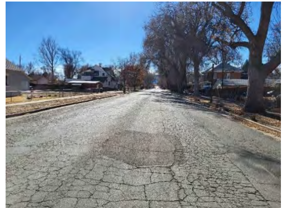
6 Alligator cracking at Robinson and 4th St.
