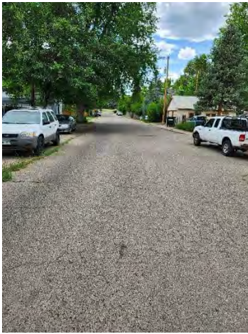
Photo 119: Hawkins Ave. south of W 3 rd St.
