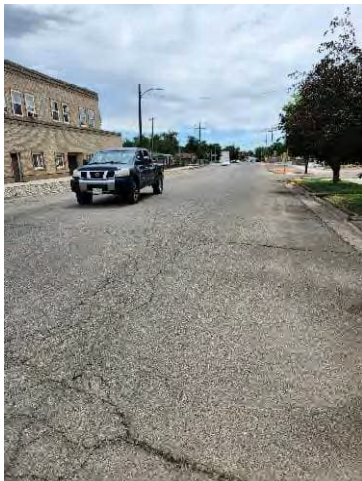
Photo 34: W Main St – west of Green St.
