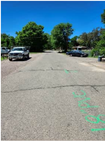
Photo 1: Teller Ave south of W. 4 th St.
