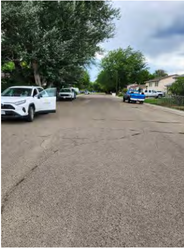
Photo 150: Robin Rd. north of E 3 rd St.
