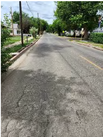
Photo 25: N Frazier Avenue, East of W 1 st Street by Intersection
