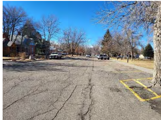
8 Poor pavement condition near the park
