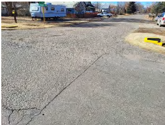
7 Transition between 2 pavement conditions
