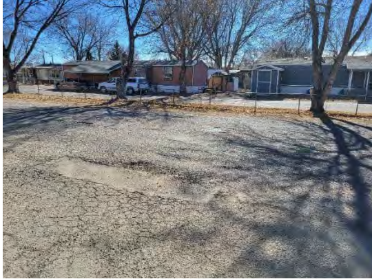
1 Road damage at Tanner Ave and 3rd St
