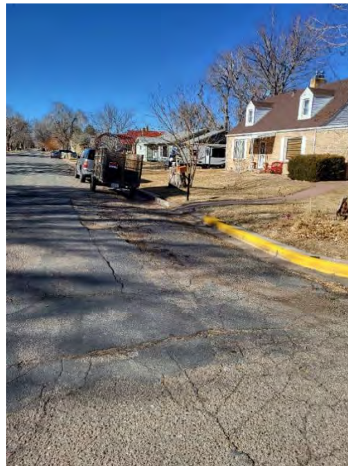
4 4th St- localized severe pavement damage.
