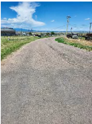
Photo 25: Moore Dr pavement transition north of Indian Hills Rd
