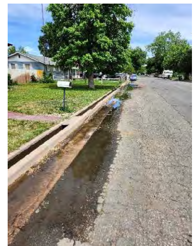
Photo 72: north edge of E 4 th St east of N McCandless Ave.
