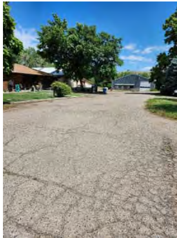
Photo 26: N Petroleum Ave north of E 7 th St (Northview)
